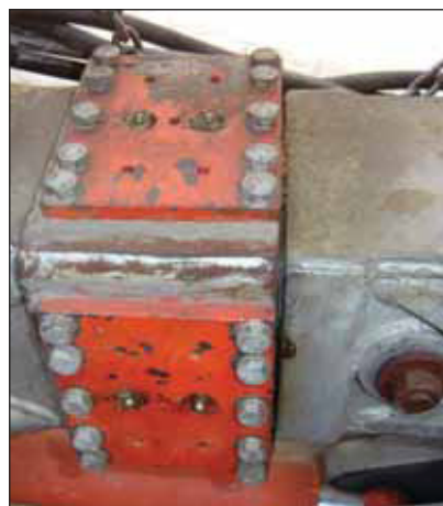
Where hot dip galvanized fasteners were used the comparison to uncoated fasteners is clearly evident.
