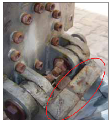
Steel components, added after hot dip galvanizing were silver painted, again illustrating the corrosive effect relative to the hot dip galvanized surfaces.
